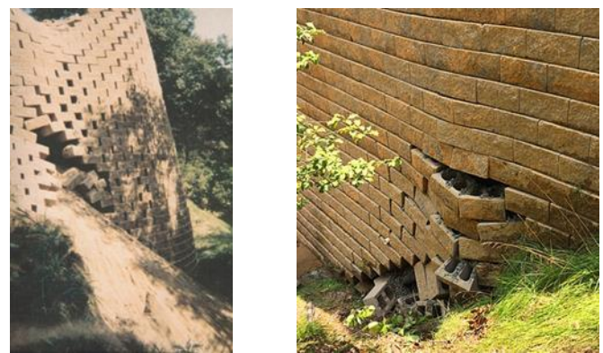
Figure 3. Toe failures of MSE walls caused by hydrostatic pressures. (compl. of Wikipedia and Google)
