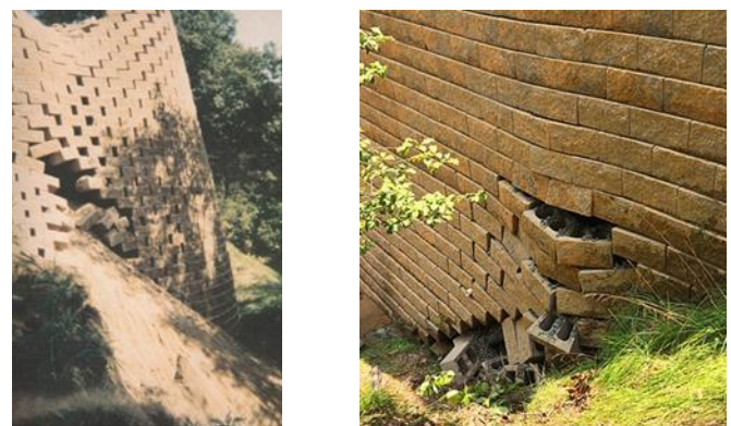
Figure 3. Toe failures of MSE walls caused by hydrostatic pressures. (compl. of Wikipedia and Google)
