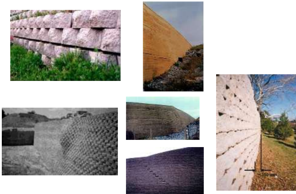
(a) Cases of Excessive Deformation
