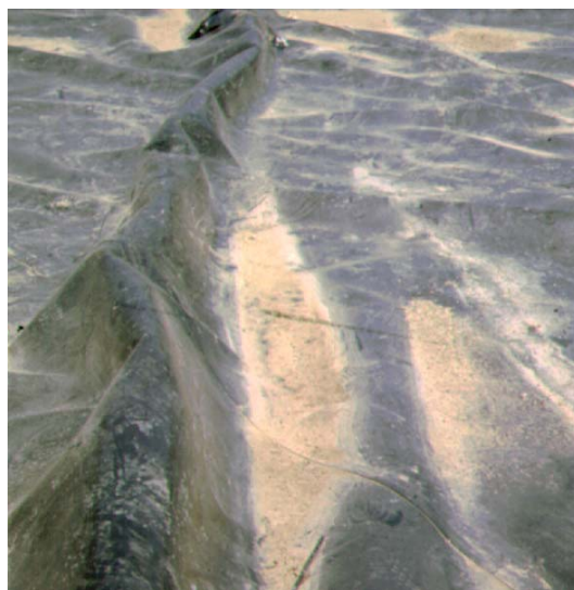
Figure 8 - Waves in HDPE geomembrane on the relatively flat base of a landfill.
