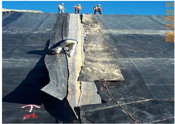
(b) Separation of GCL panels \approx 200 mm (8 in.) (California, 2004)
